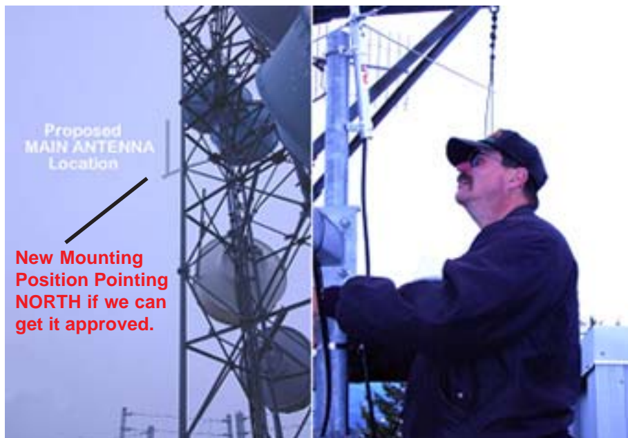
Gary, KE7IAT finishing back-up antenna installation on a cold day in September.
